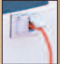
Outside electrical receptacle
